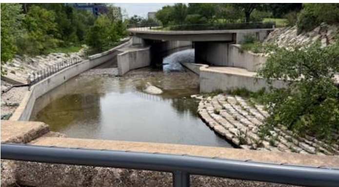
Pond area adjacent to the Waller Creek Tunnel inlet. Considerable debris gathers in this channel after storm events
